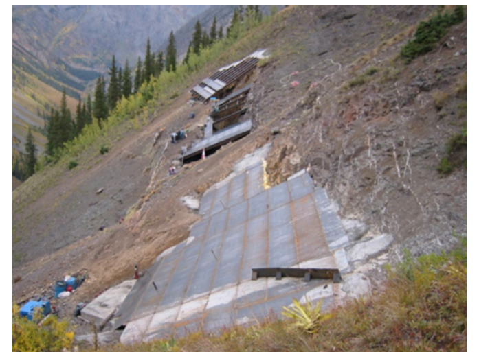
Large stope closures, San Juan County, CO.
