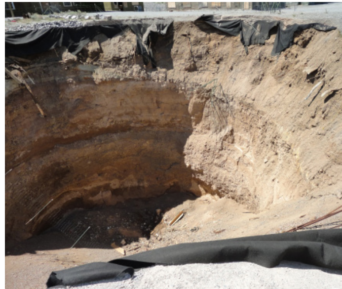
Subsidence of the Chief No. 1 shaft. Note the unconsolidated waste rock and native soil that has sloughed into the 1,800-ft deep shaft accessing extensive mine workings. The frayed geotextile and crushed limestone of the engineered cap can be seen on top.
